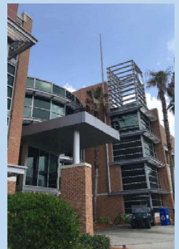
Figure 3. Existing Architectural Detailing
