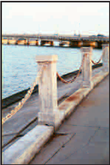
Aging post and chain railing system along bulkhead
