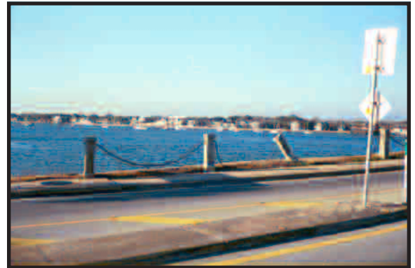
Aging concrete post and chain railing system
