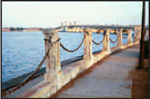
Cracked and rusted railing system
