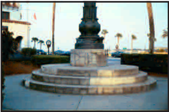
Cracked concrete base of flagpole
