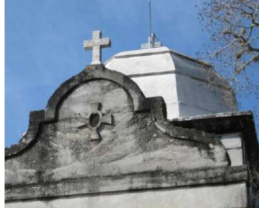
The eastern face was repaired with concrete decades ago, which is now falling apart.
