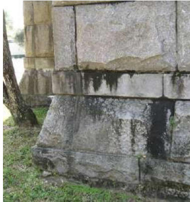
Granite needs cleaning & repointing.
