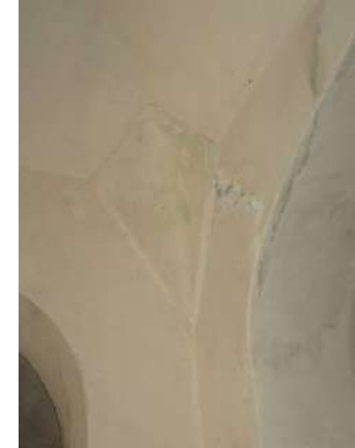
Water and moisture damage inside of the mausoleum.
